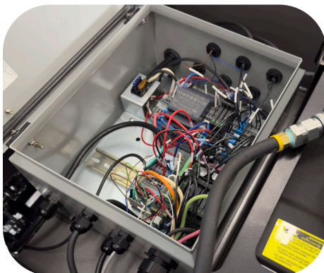
Larger Accessible Electrical Box
